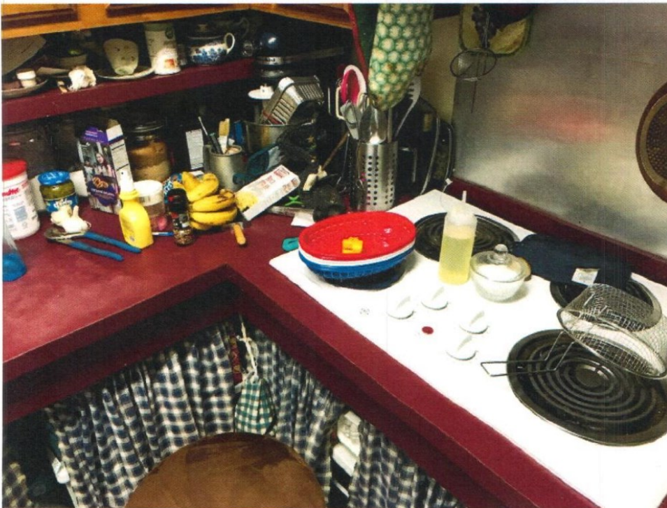
COUNTER TOPS IN POOR CONDITION
