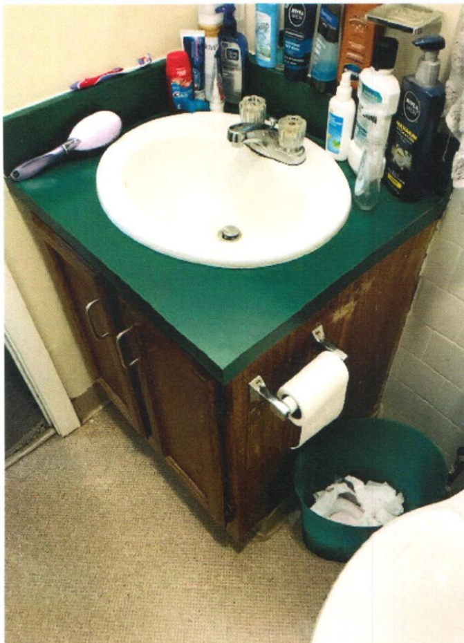
VANITIES IN POOR OVERALL CONDITION
