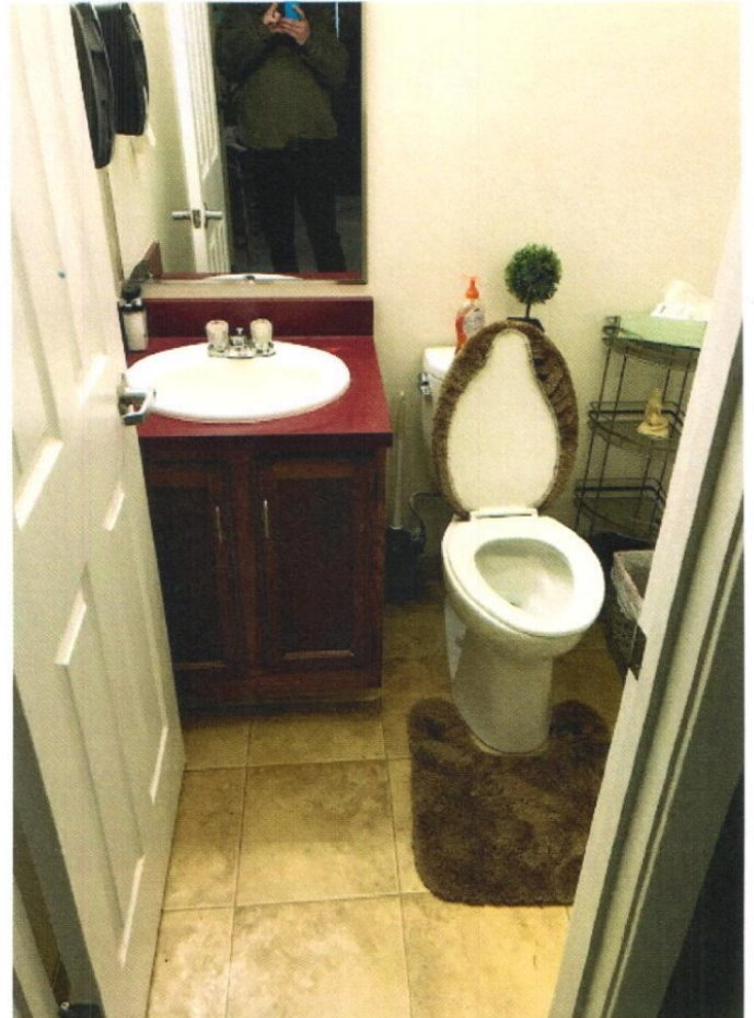
TYPICAL FIRST FLOOR HALF BATH REQUIRING UPDATES
