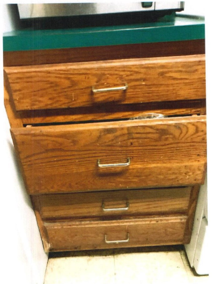
CABINETS IN POOR CONDITION
