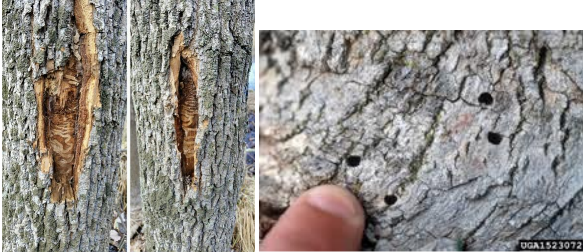
Specific signs of the emerald ash borer: (left) larval "tunnels" damage to cambium layer under bark; (right) D-shaped exit holes in bark.
