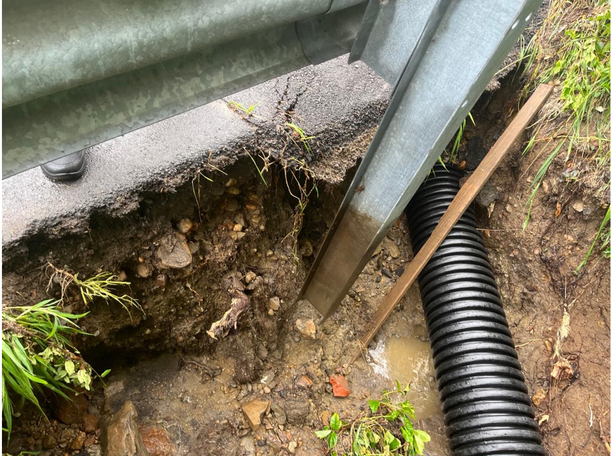
Undermined section of the sidewalk 322 Main Street. Area of sidewalk has been closed by local and State DOT.
