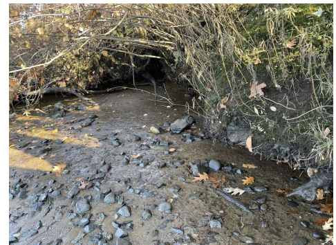
Erosion undermining bank
