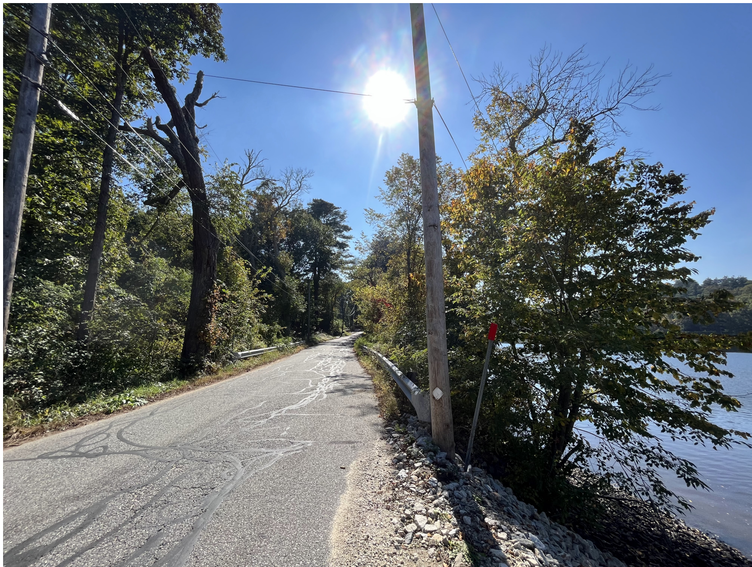
View of crossing looking west on River Road. Note the support utility pole within inches of the eroded river bank. 10/5/2023
