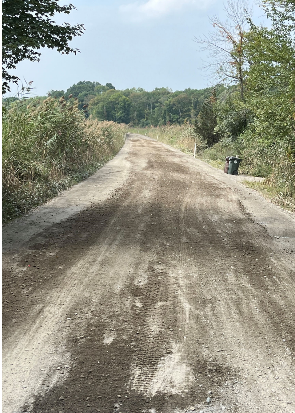
Completed work viewed looking northwest from end of gravel road at southeast connection to paved road
