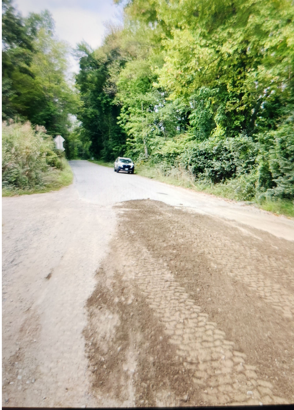
Existing Condition Photo 2: Gravel road meets paved road looking northwest. Area that appears "disturbed" is freshly spread gravel from 9/8/2023 emergency work.
