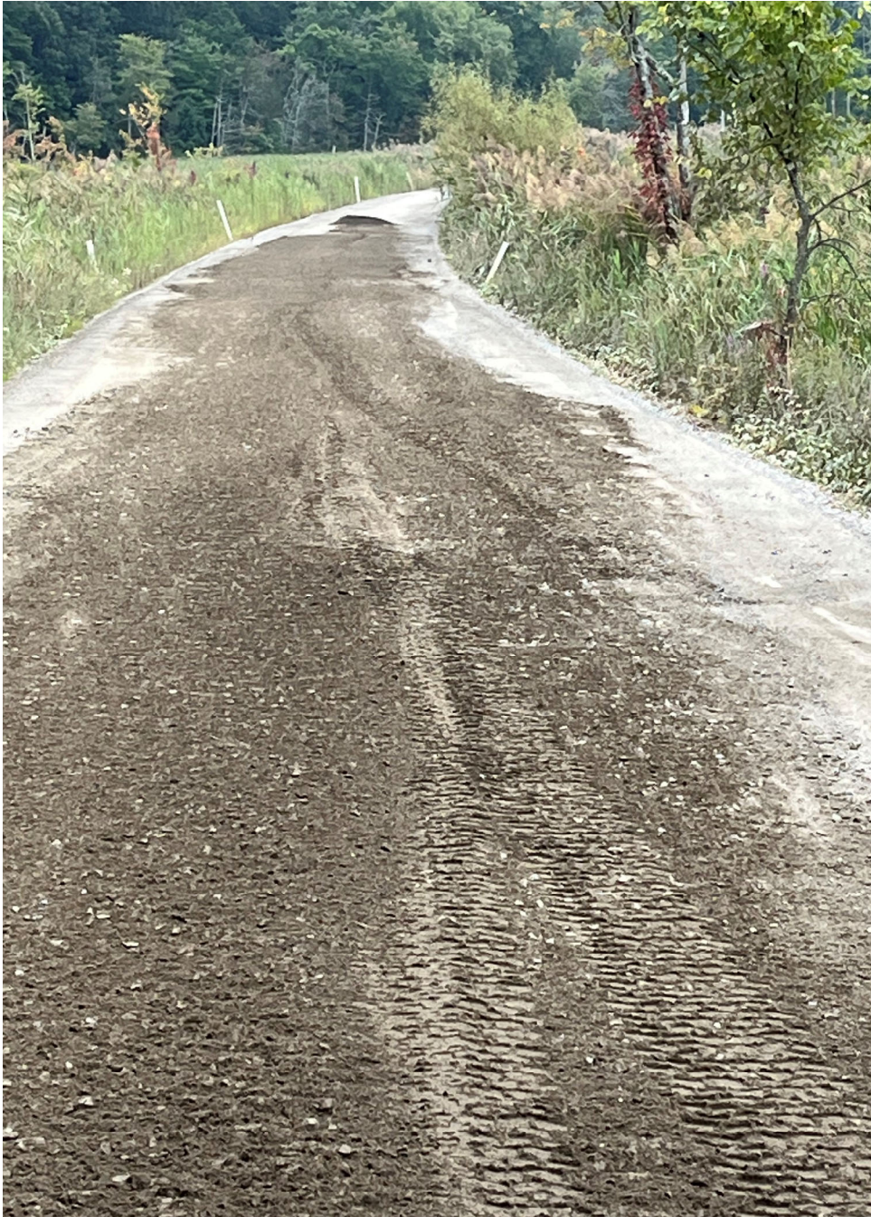
Looking southeast at material spread to be compacted and a pile of material to spread
