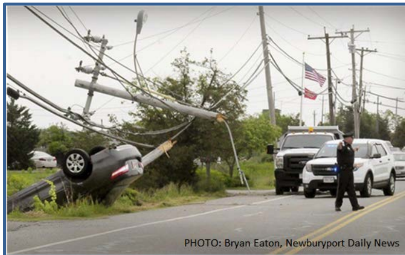
Figure 54. Turnpike Accident - Shuts off power to 1310 Plum Island Homes for 6 Hours
