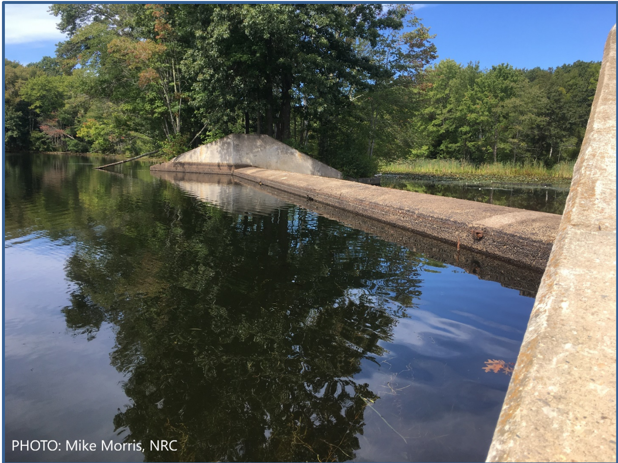
Figure 25. Low Water Level Vulnerability - Rear of Lower Artichoke Spillway September 5, 2019
