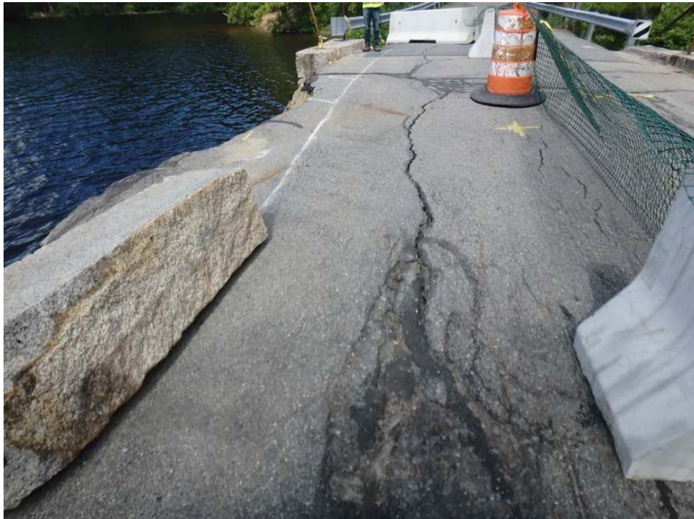
SETTLEMENT AND COLLAPSING ROADWAY
