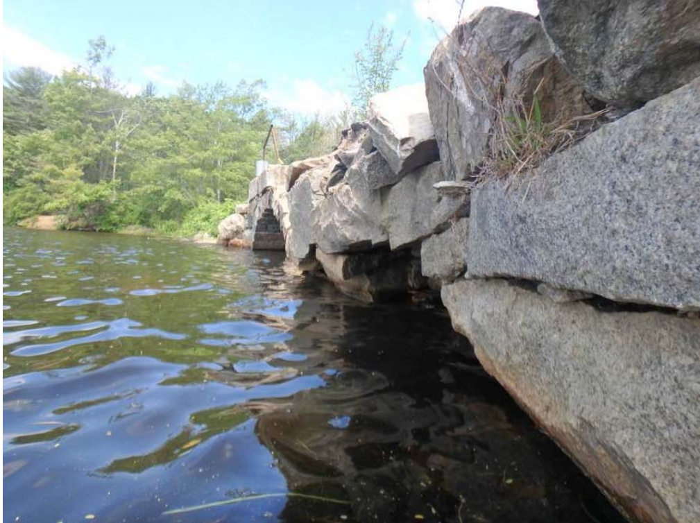
SOUTHEAST WINGWALL DISPLACEMENT
