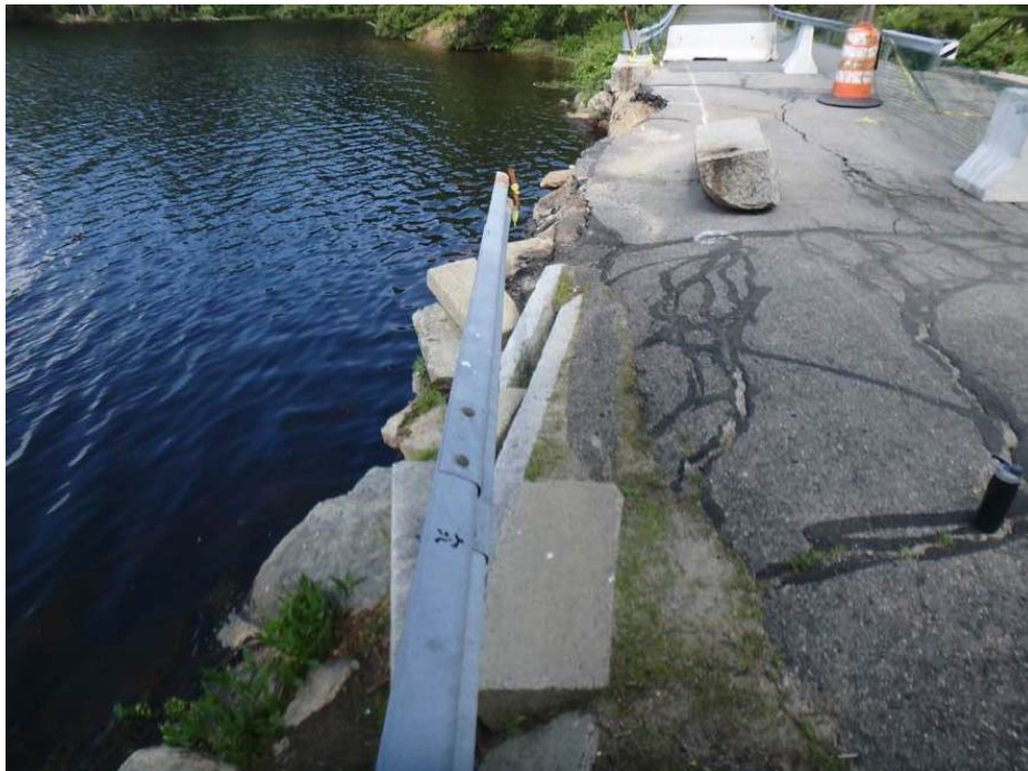
COLLAPSED ROADWAY AND SPANDREL WALL
