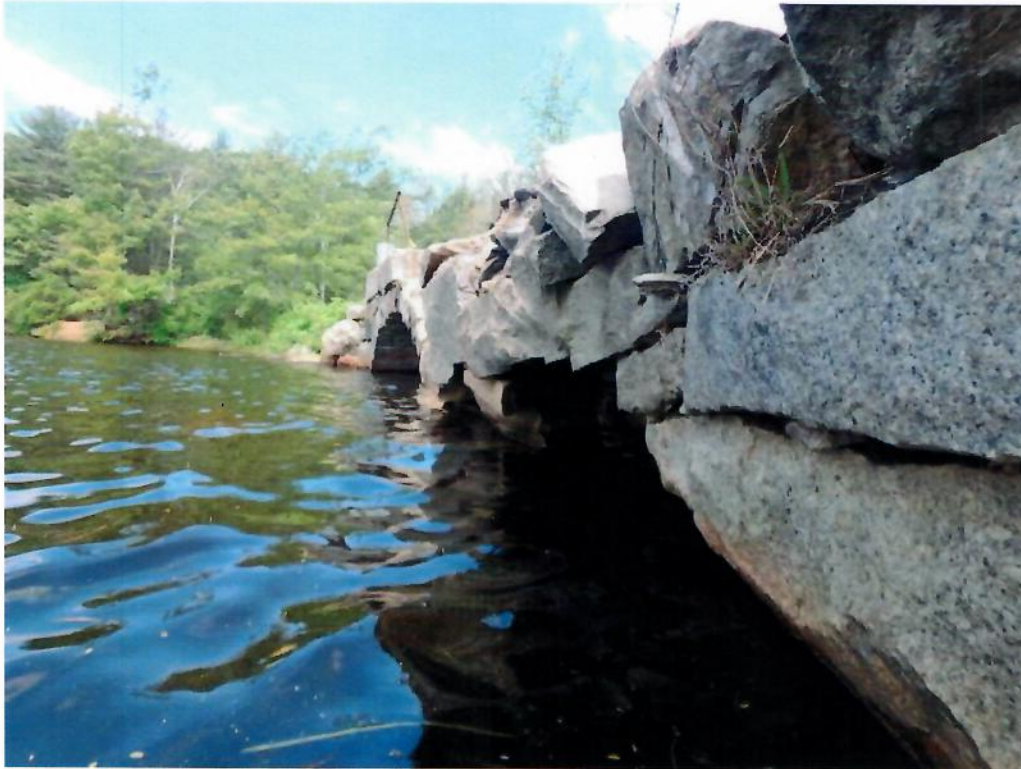
Photo 5: Severe southeast wingwall displacement.
