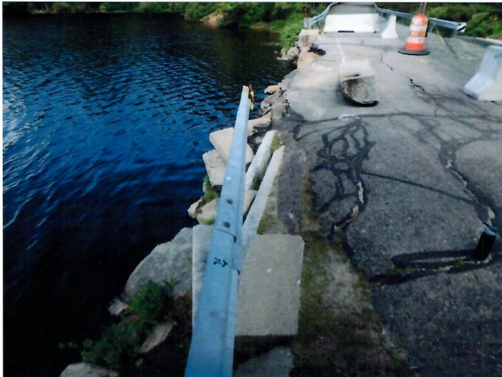
Photo 2: Failure of the spandrel wall at the southeast corner of the bridge.
