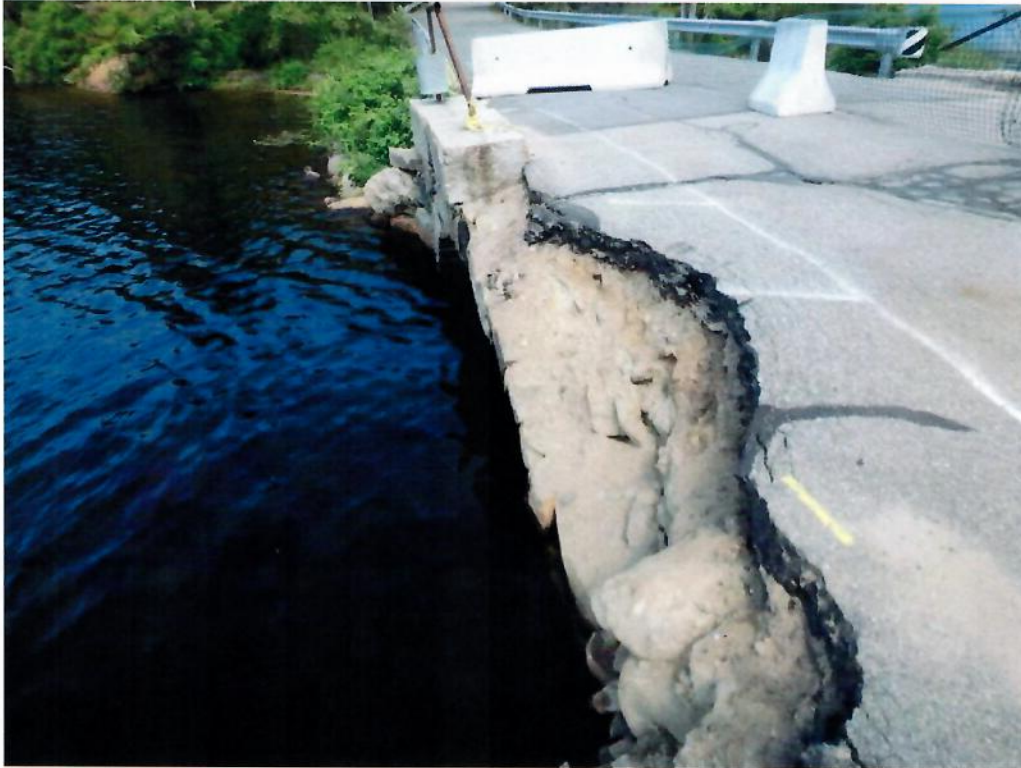
Photo 3: Failure of the spandrel wall at the southeast corner of the bridge.
