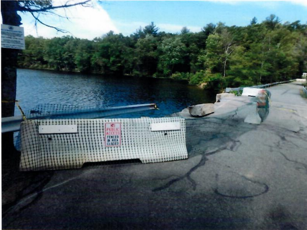
Photo 1: Jersey barriers with construction/snow fencing blocking off the failure of the spandrel wall at the southeast corner of the bridge.
