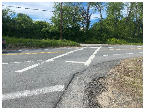
Image 1: Skewed/Faded Crosswalk at the Pipestave Recreation Area Driveway
