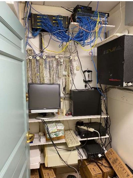
The existing phone system is antiquated, and its hub is located in a publicly-accessible location (mail room), presenting a security risk.
