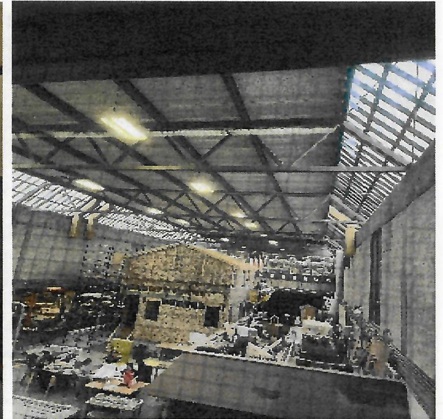
Glazed opening contain wire glass that is not impact rated /no longer to code
