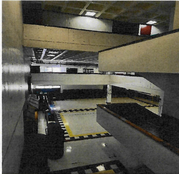
Multiple atria connect floors lacking code required separation or sprinkler & smoke protection systems
