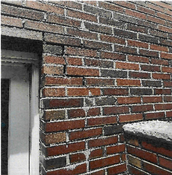
Brick construction doesn't meet current energy codes & needs repair, roofs & windows past serviceable life
