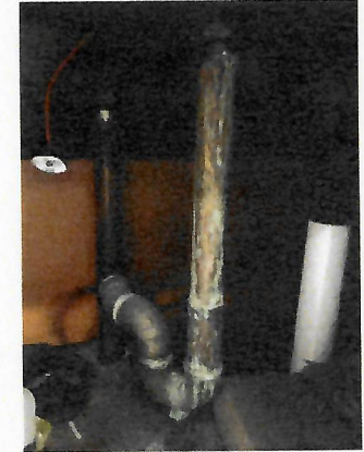
Non-compliant Lab piping
