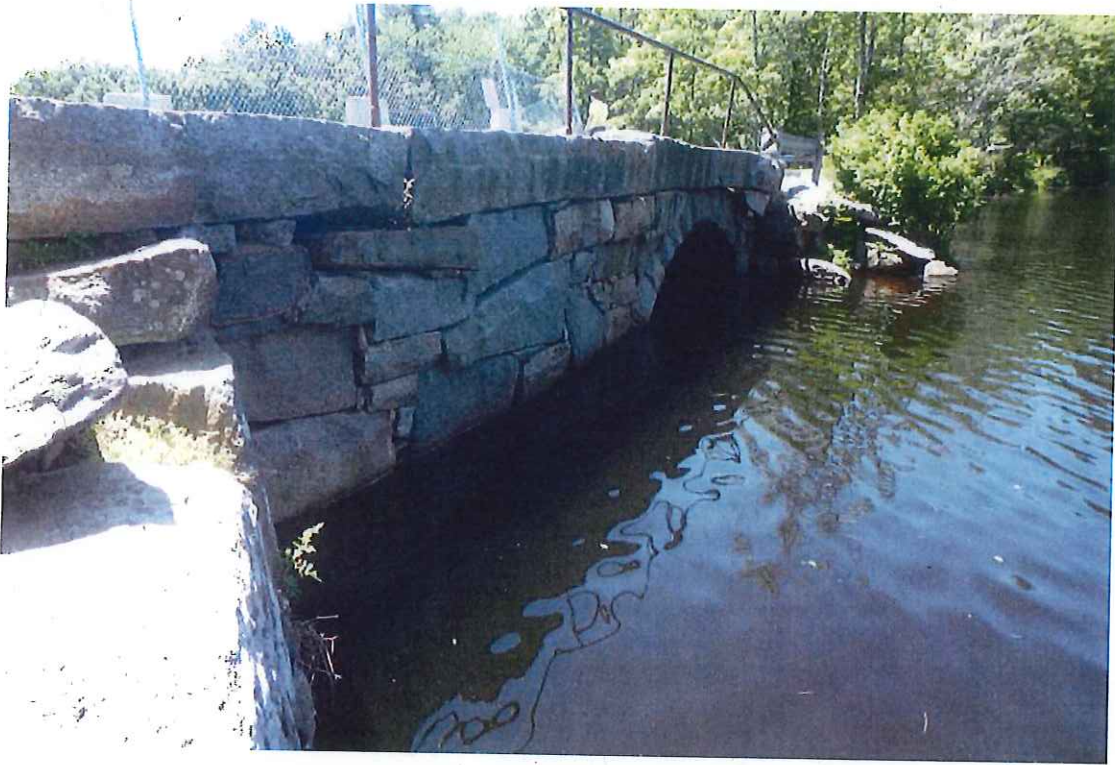
Photo 9: Bulging of the north spandrel wall both east and west of the arch.
