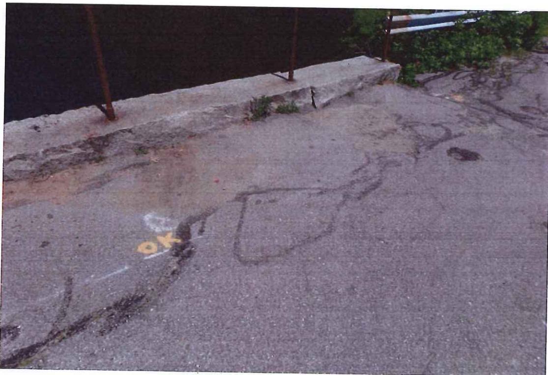
Photo 8: Settlement areas adjacent to the north bridge railing.
