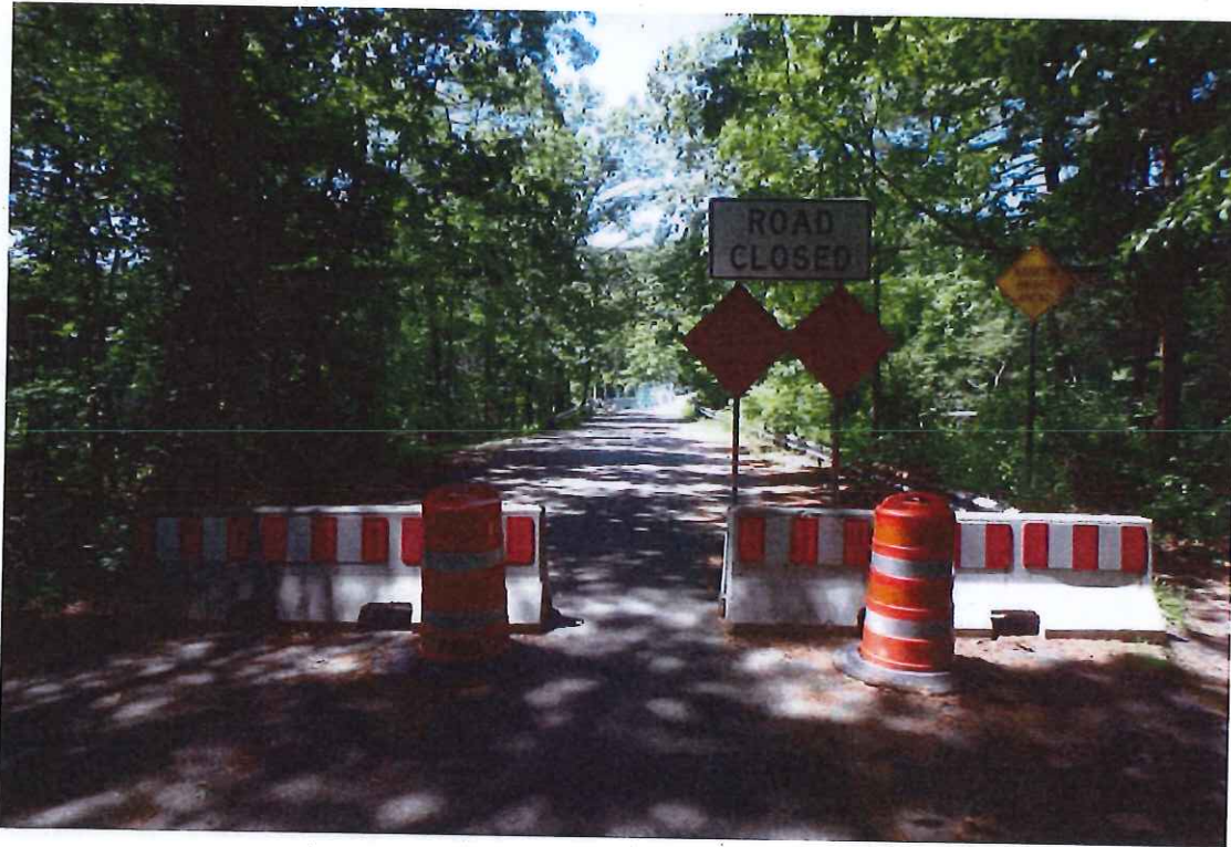
Photo 7: Typical barrier and signage at bridge preventing vehicular traffic. East approach shown.
