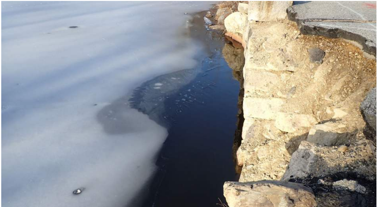
Photo #4: View northwest of Plummer Spring Rd, Newburyport facing Middle St, West Newbury over the Upper Artichoke Reservoir.. Up close view of the bridge in disrepair.
