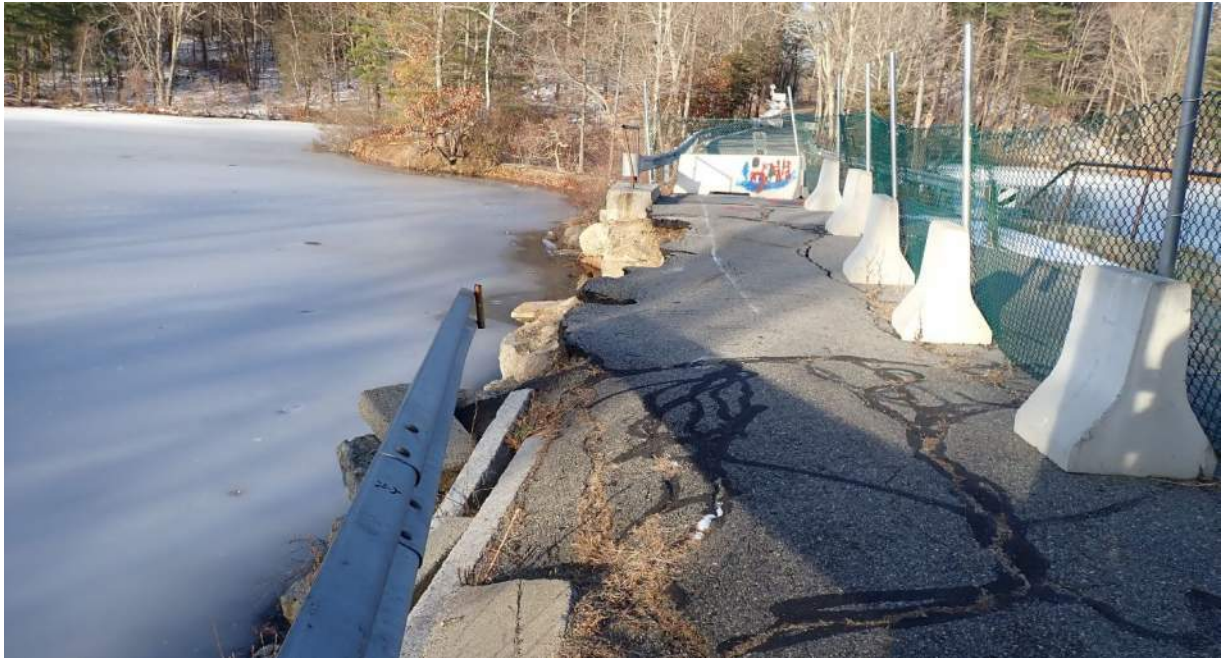
Photo #3: View northwest of Plummer Spring Rd, Newburyport facing Middle St, West Newbury over the Upper Artichoke Reservoir. View of the failed section at the southern end of the roadway, directly over the bridge which is closed for public safety.
