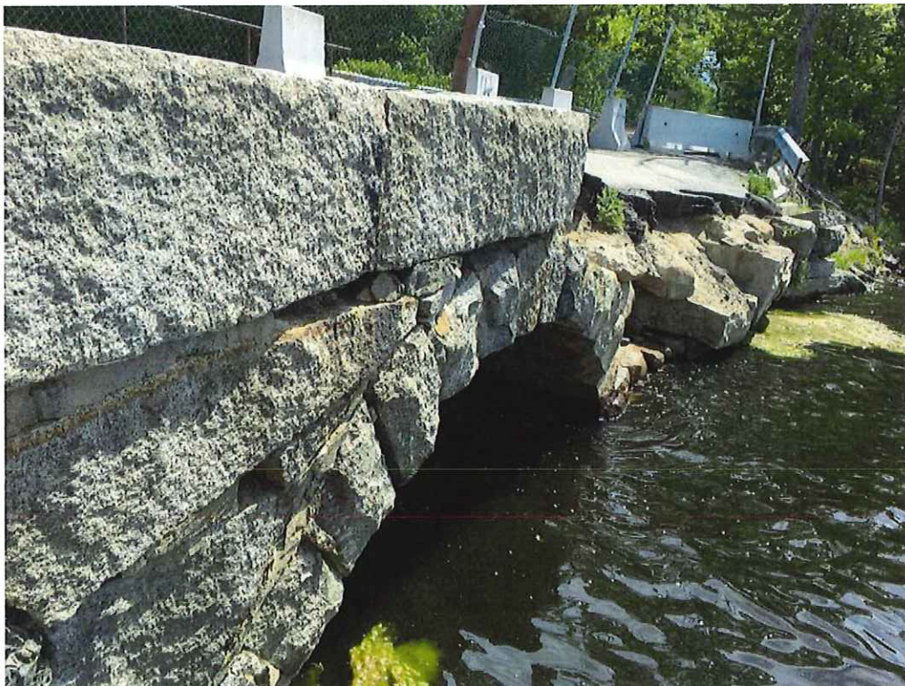
Photo 16: The collapsed spandrel wall along the south side of the bridge.
