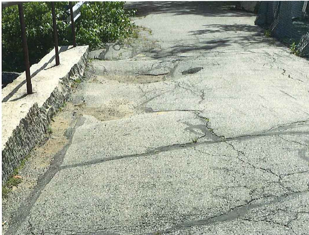
Photo 10: Areas of heavy settlement and depression along the north spandrel wall (heaviest at the East end) up to 1' deep. (Looking East).
