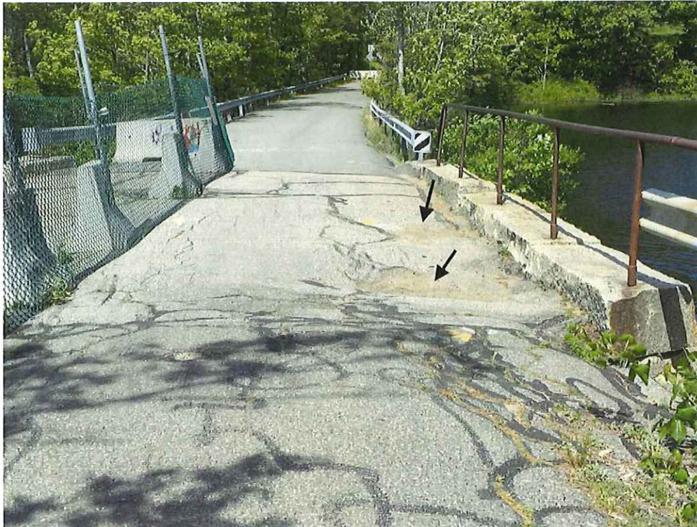
Photo 11: Areas of heavy settlement and depression along the north spandrel wall (heaviest at the East end) up to 1' deep. (Looking West).
