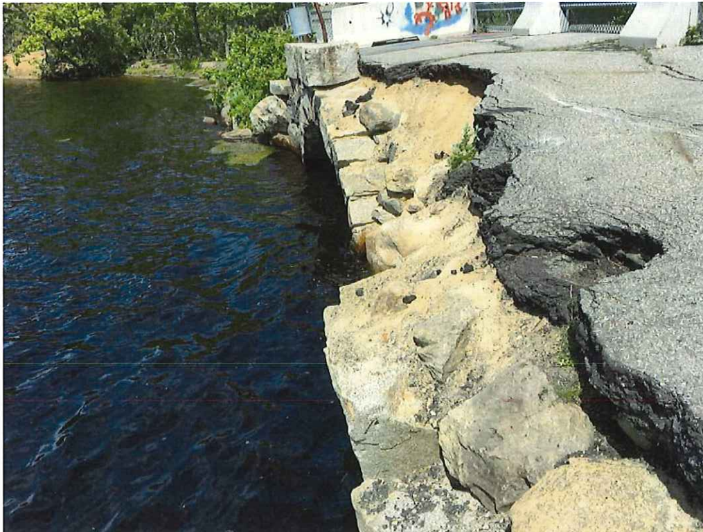
Photo 14: The collapsed area along the south side of the bridge and signs of the progression of the washout. (Looking West).
