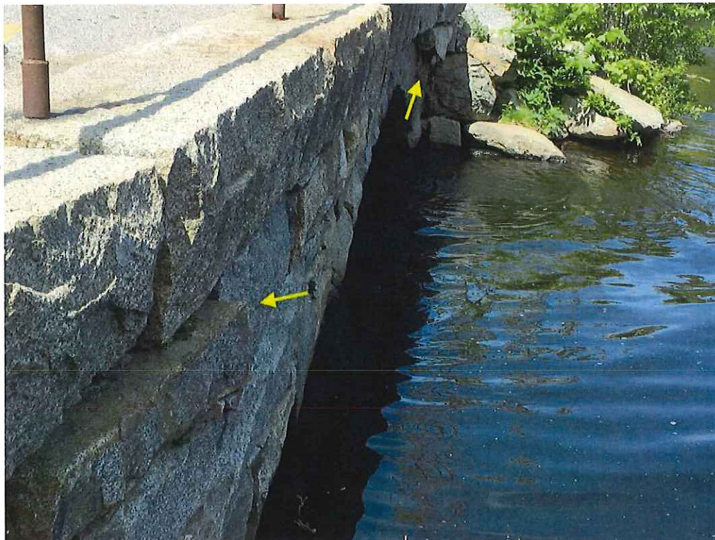
Photo 12: North spandrel wall, outward displacement mostly along the top course and cap stones, up to 5".
