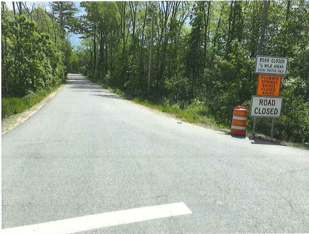
Photo 1: First advanced, "Road Closed Ahead" signs, west of the bridge.
