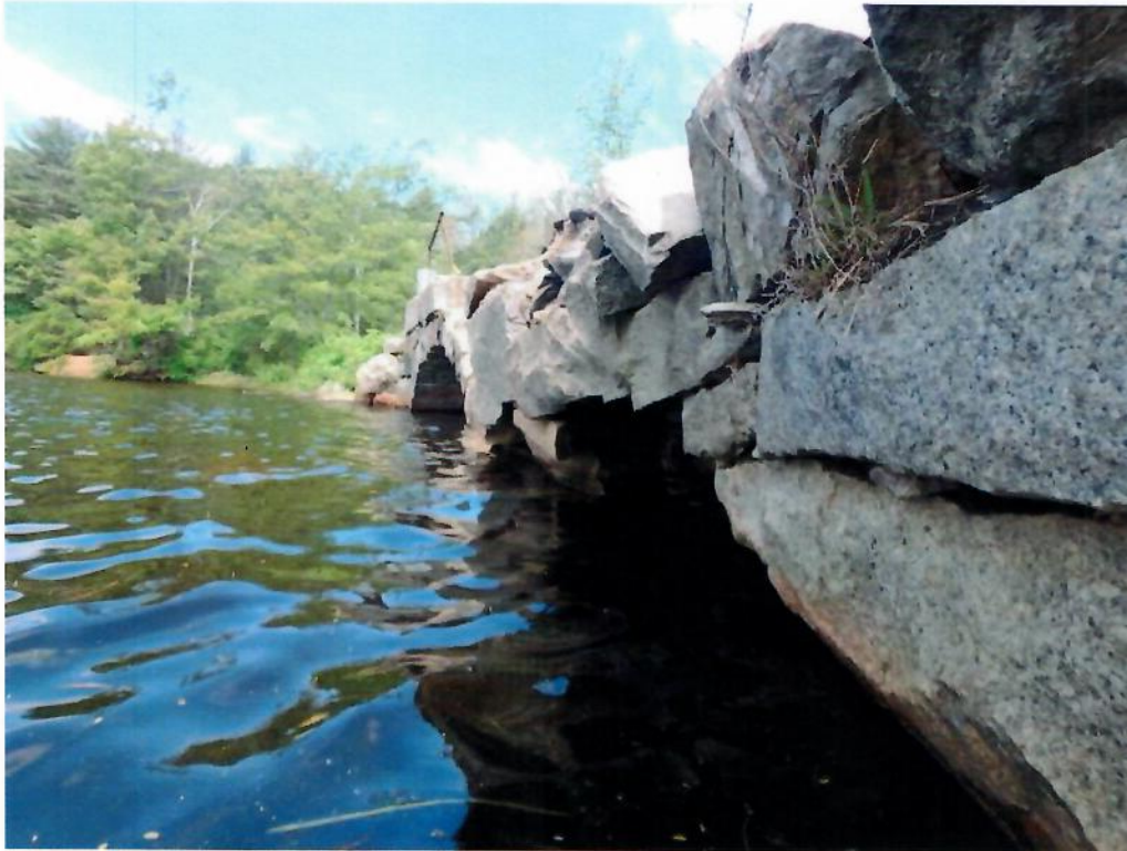
Photo 5: Severe southeast wingwall displacement.
