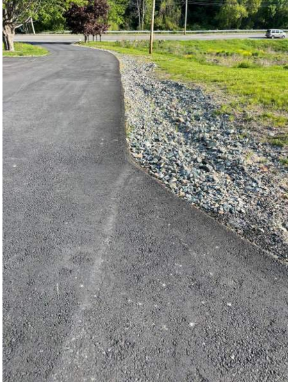
Common Drive – Rip Rap Swale – North Side
