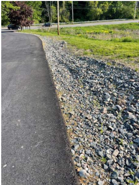
Common Drive – Rip Rap Swale – North Side
