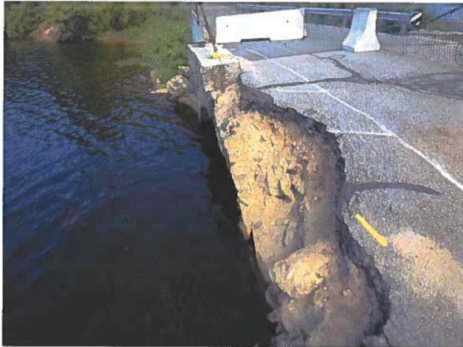
COLLAPSED SPANDREL WALL
