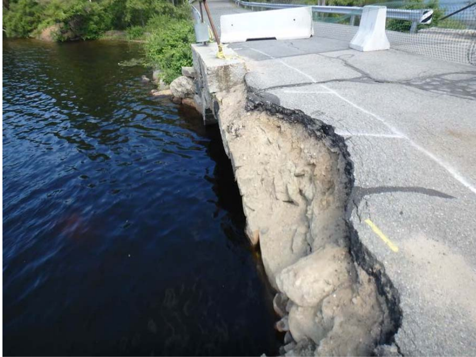
COLLAPSED SPANDREL WALL
