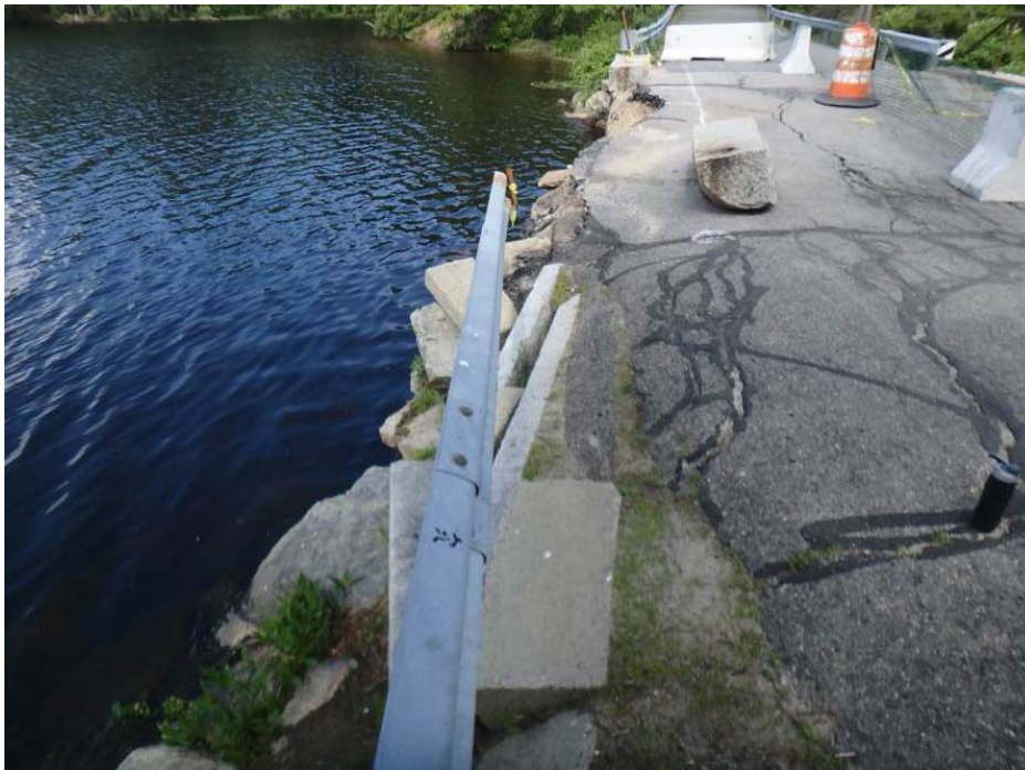
COLLAPSED ROADWAY AND SPANDREL WALL
