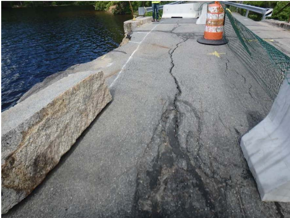
SETTLEMENT AND COLLAPSING ROADWAY
