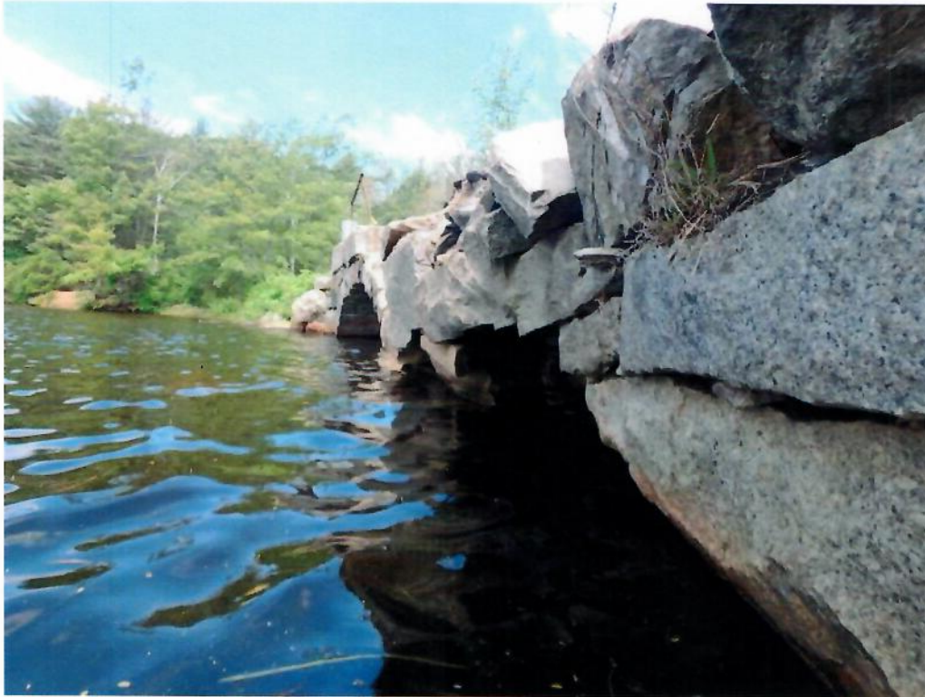
Photo 5: Severe southeast wingwall displacement.
