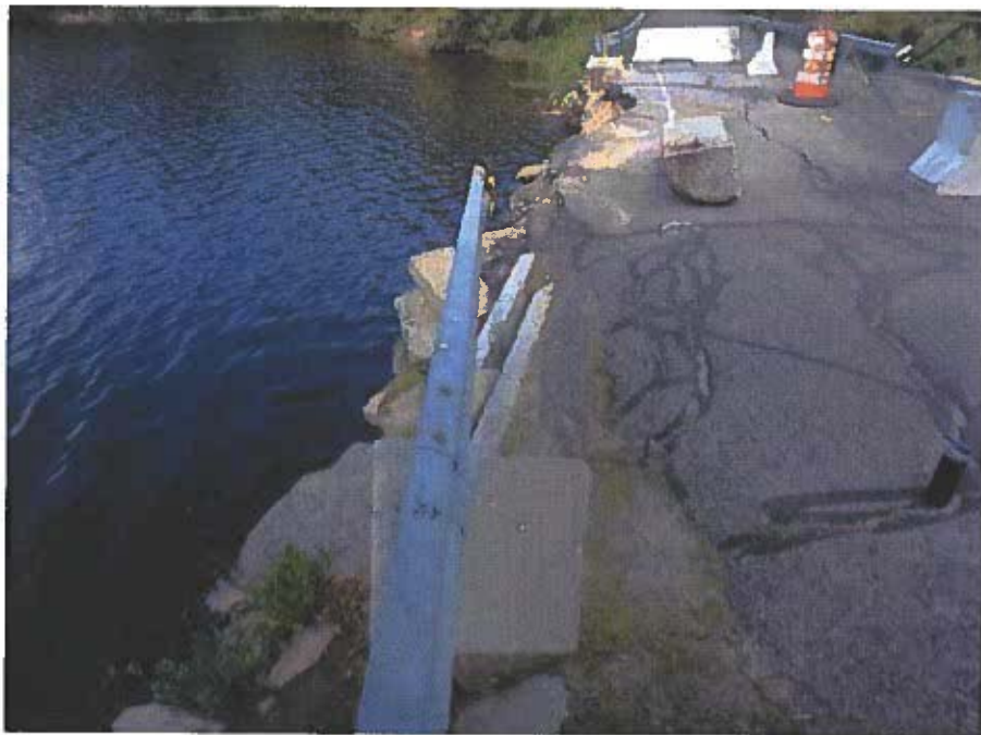
COLLAPSED ROADWAY AND SPANDREL WALL
