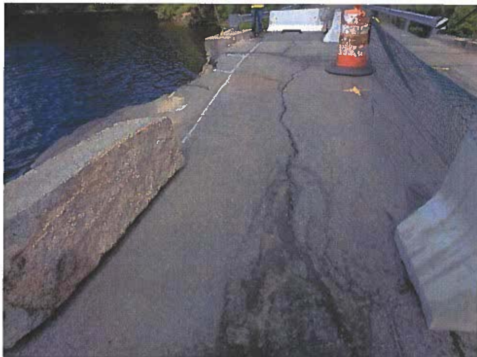
SETTLEMENT AND COLLAPSING ROADWAY
